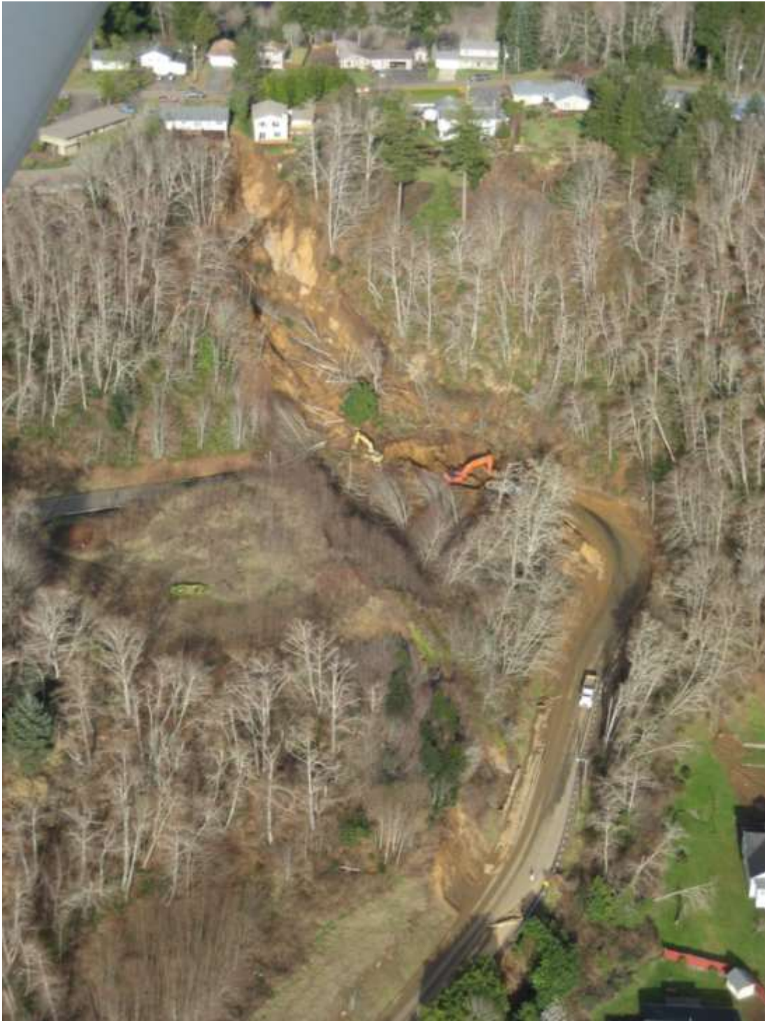
Figure 9-8 Aerial image of January 2015 landslide blocking Beacon Hill Drive Source: Washington Department of Natural Resource
