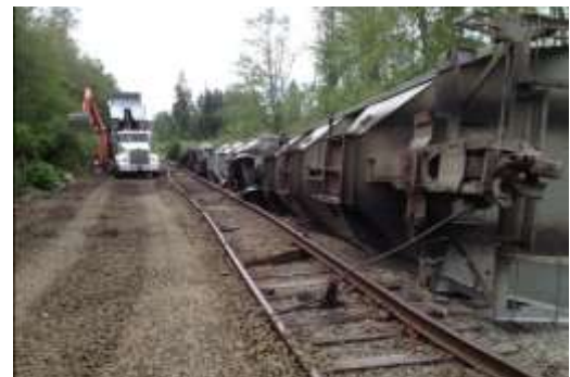
Figure 14-6 Derailed Train Cars - Montesano May 15, 2014
