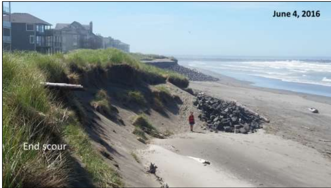
Figure 7-21 End Scour North of the Ocean Shores Rock Revetment
